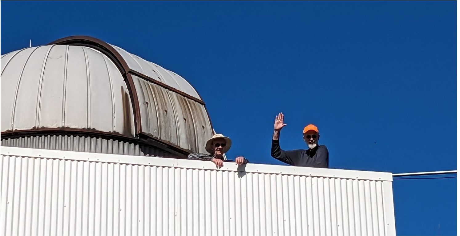
Jeff KB1LZ and Sam W1SMF install lanyards and pulleys for wire antennas
